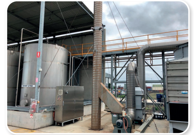
Stack Emission Testing Ports at Australian Agribusiness Lara site
