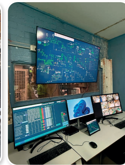
SCADA System for monitoring the salt refining process
